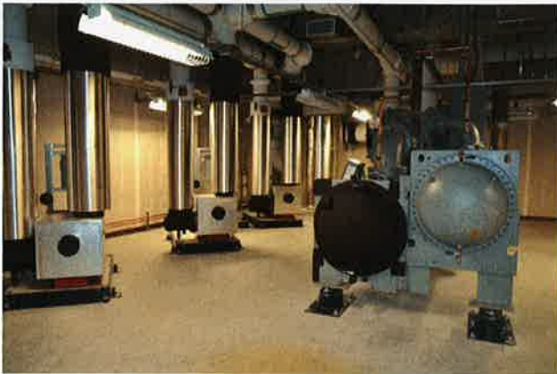
The chilled-water plant at Mills-Peninsula Medical Center.
