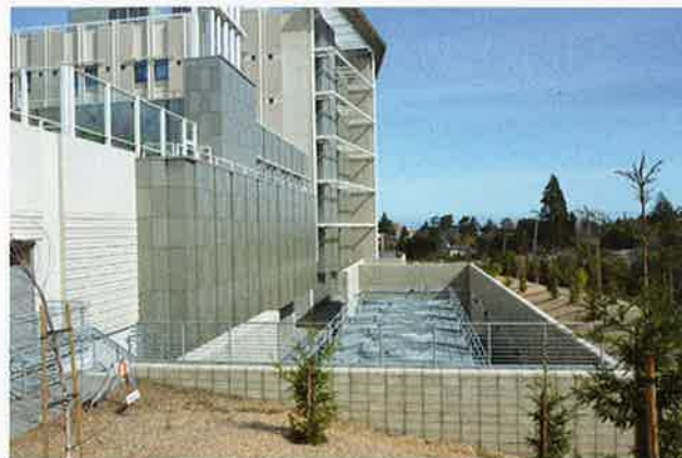
Cooling towers in the service yard. Note their proximity to a nearby residential area.
